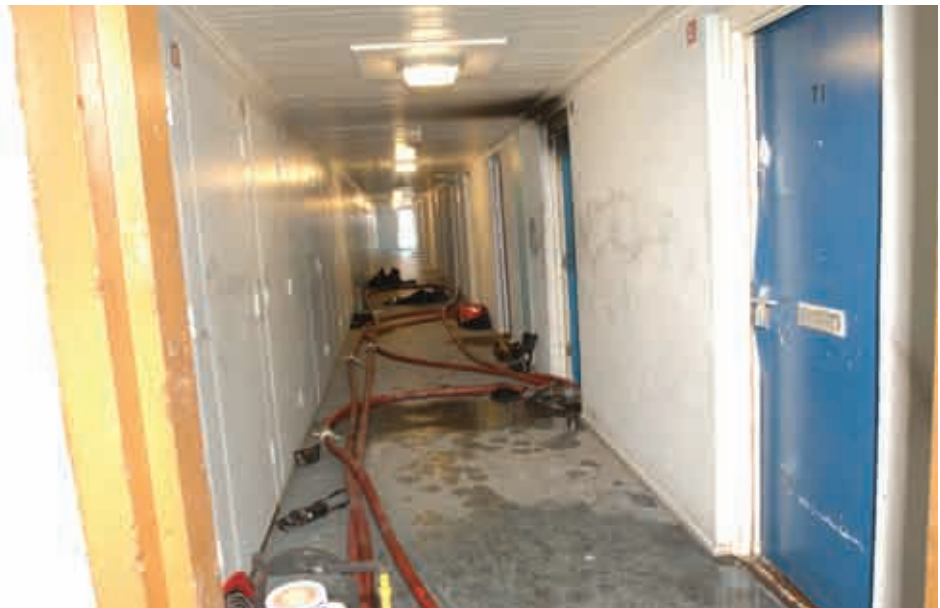
Fig 16: Post incident photograph of ninth floor. The second door on the right is the entrance to Flat 72. The white panel doors on the left are the fire escape doors to other flats. Note the relatively minor smoke damage. (Source: Hampshire Constabulary)
