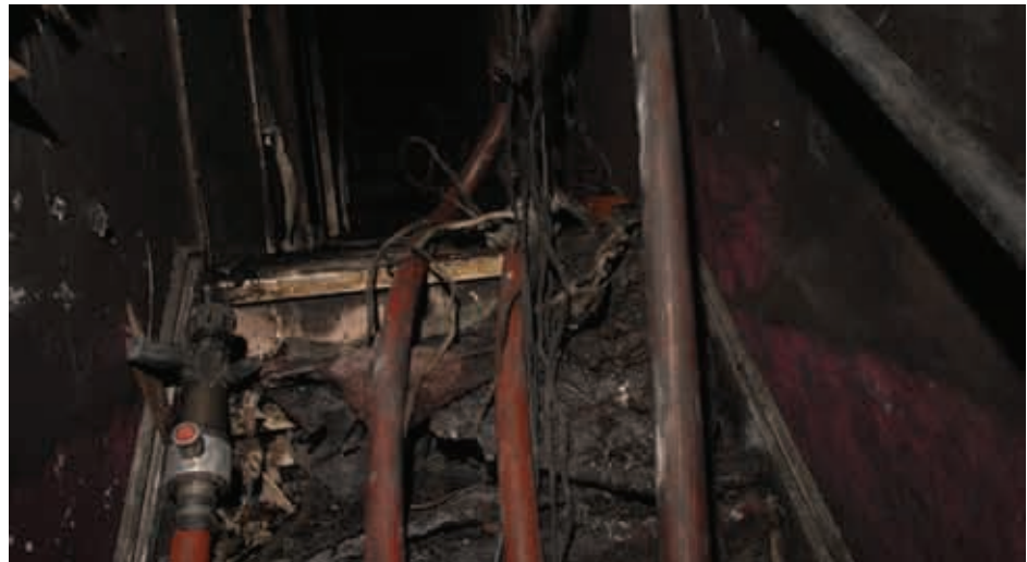
Fig 23: Post incident photograph looking up stairs from lounge window towards bathroom level. (Source: Hampshire Constabulary)
