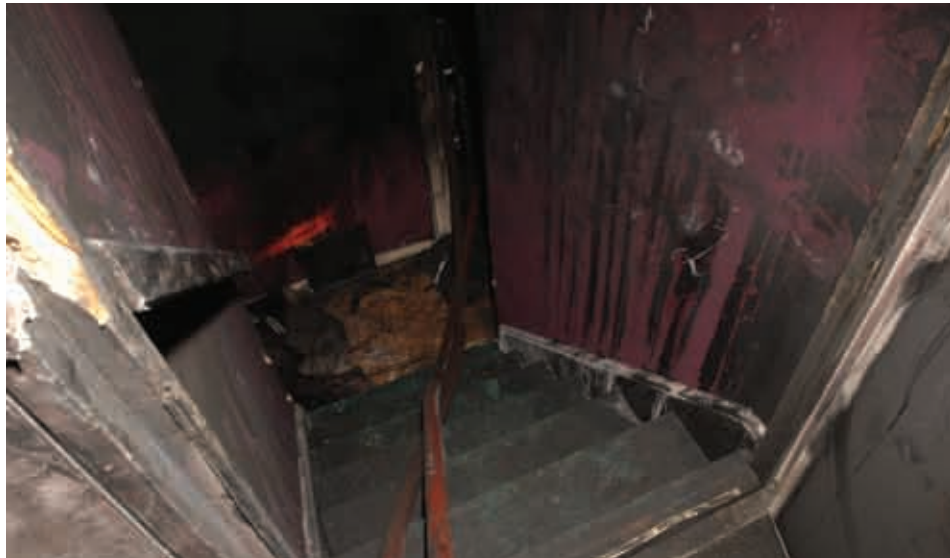
Fig 28: Post incident photograph from eleventh floor fire escape door down staircase to bedroom floor level (Source: Hampshire Constabulary)
