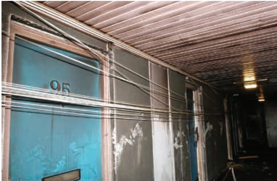
Fig 31: Post incident photograph of the eleventh floor landing showing displaced cables (Source: Hampshire Constabulary)
