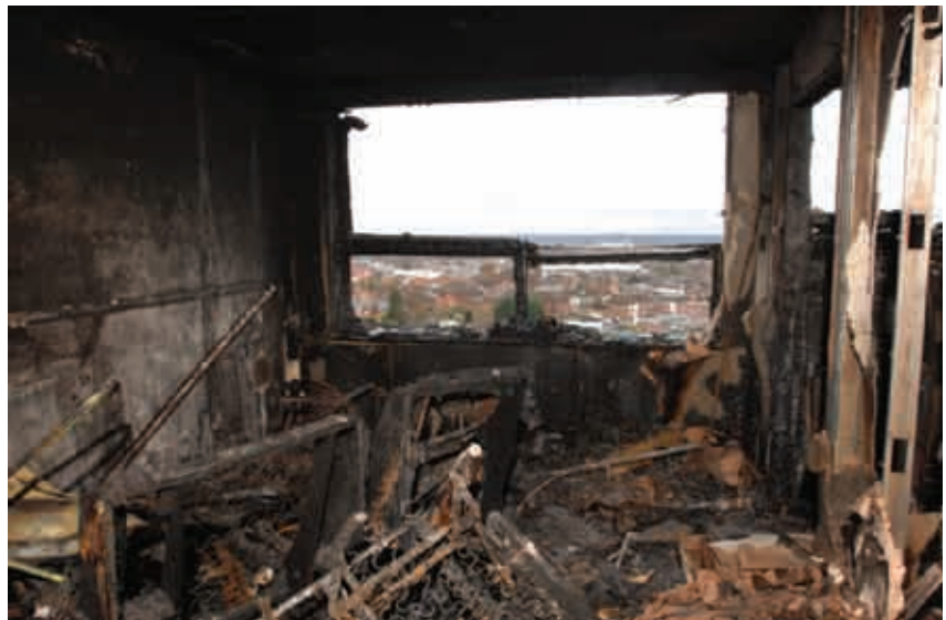
Fig 36: Post incident photograph from top of entrance stairs towards lounge window. (Source: Hampshire Constabulary)
