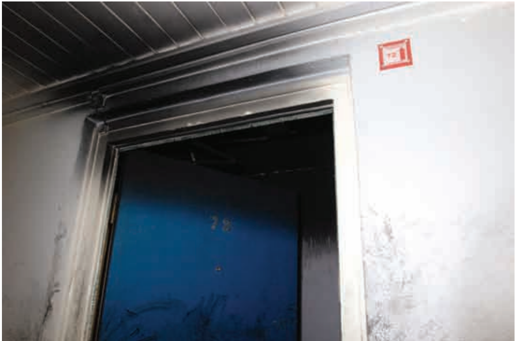
Fig 10: Post incident photograph of flat sign denoting (by arrow) that Flat 72 is an 'up' flat. Note the relatively minor smoke damage (Source: Hampshire Constabulary)
