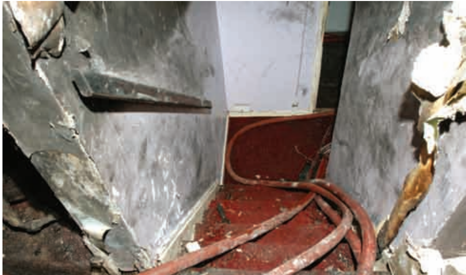
Fig 18: Post incident photograph from lounge level down stairs to entrance lobby. (Source: Hampshire Constabulary)
