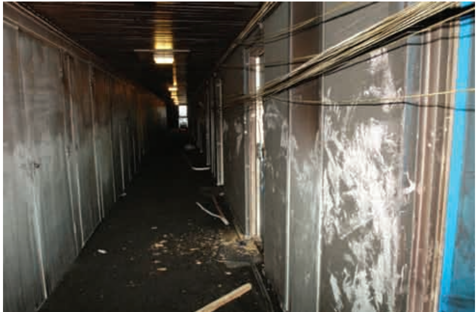
Fig 30: Post incident photograph showing conditions on the eleventh floor after the escape door from Flat 72 was left open. Note the displaced cables. (Source: Hampshire Constabulary)
