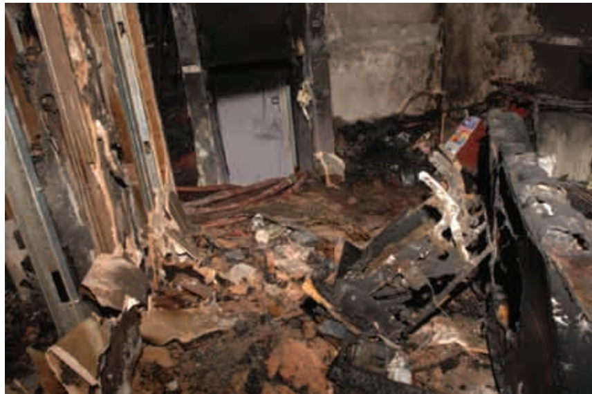
Fig 35: Post incident photograph of lounge from the window back towards staircase from entrance (middle) and the stairs leading up to the bedrooms (left hand side). (Source: Hampshire Constabulary)
