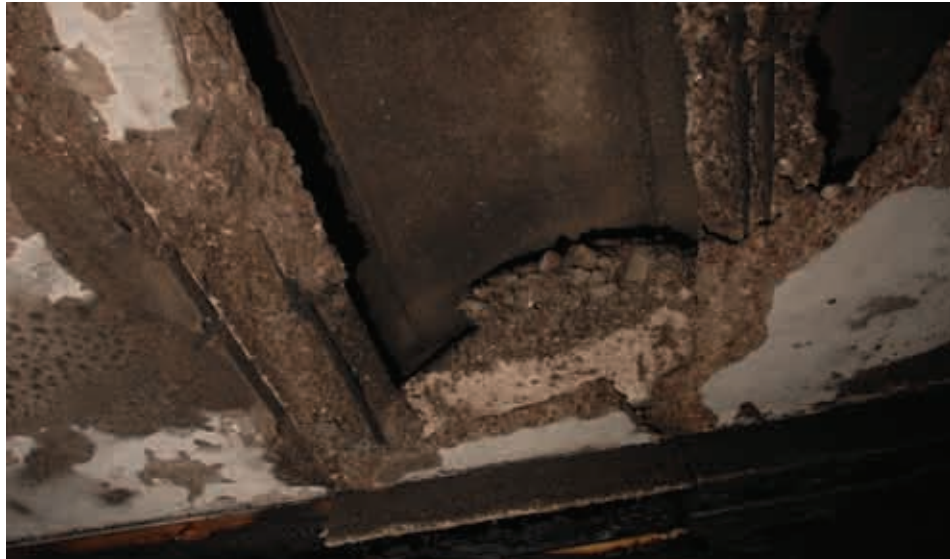
Fig 27: Post incident photograph of kitchen ceiling showing the fire damage to the concrete beams (Source: Hampshire Constabulary)
