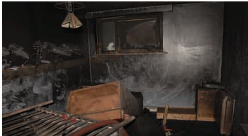
Fig 20: Post incident photograph of Bedroom 1 showing bedroom window (Source: Hampshire Constabulary)
