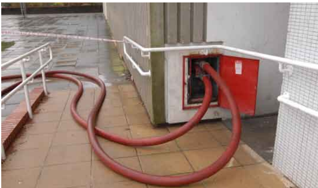
Fig 4: Post incident photograph of dry riser inlet with 2 x 70mm supply hoses connected (Source: Hampshire Constabulary)
